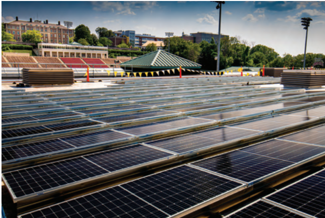
470-kilowatt rooftop solar array installed on Kirby Sports Center in 2022
