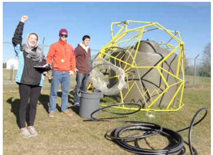
Professor David Brandes (top, center) tests and installs a solar-powered well water system for irrigation at LaFarm with students in his hydrology course; students then celebrate the system's success.
